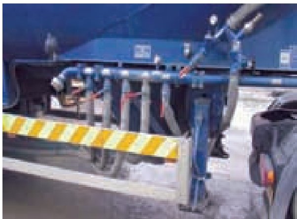
Pressure Gauges and Relief Valves
