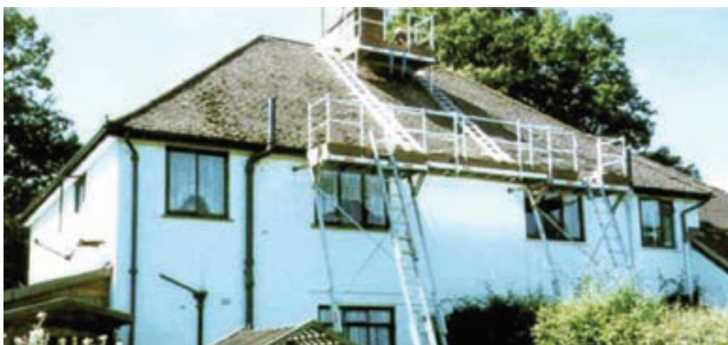
Figure 8.10: Proprietary system for access to roof and chimney.
