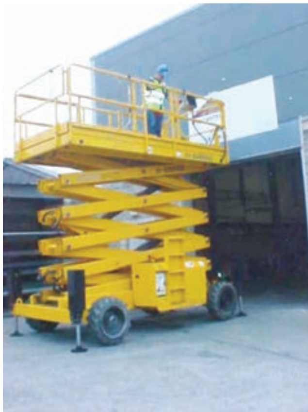
Figure 13.2: Simple mobile access used for short term work at parapet level.
