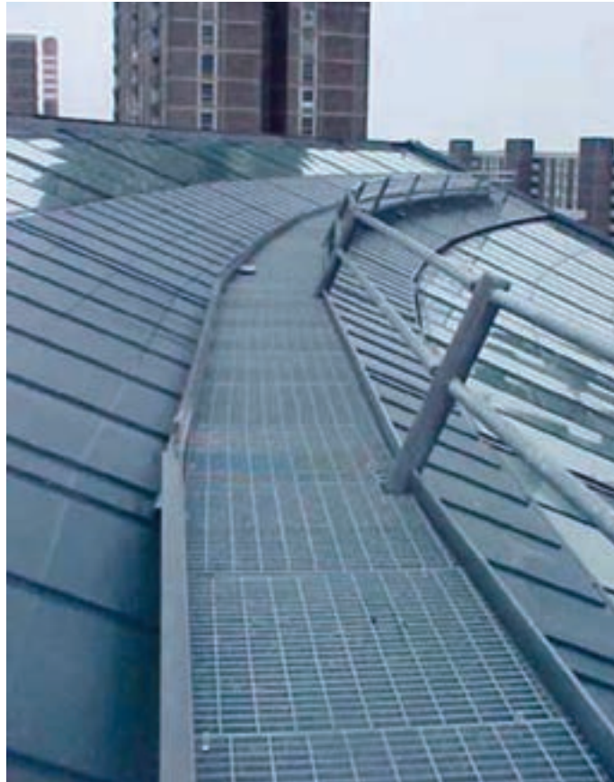
Figure 4.1: Permanent walkway giving safe access on a fragile roof. (This walkway was included in the initial design).
