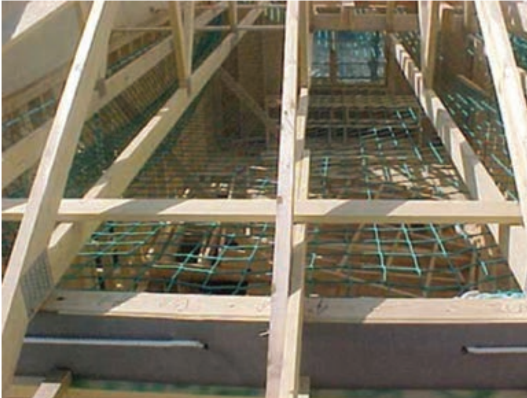
Figure 8.3: Safety nets used to give collective protection in the erection of housing roofs
