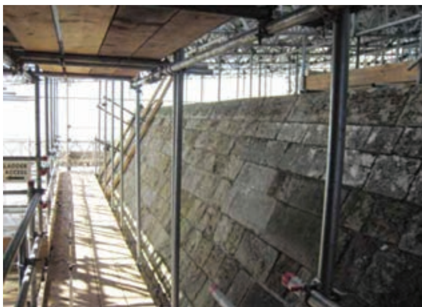
Figure 11.1 Providing safe access and a safe working platform at roof level (source Office of Public Works, National Monuments).
