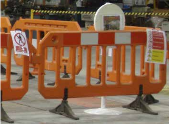
Figure 9.5 — Temporary barriers and warning signs to restrict access into strong fields generated by a temporary installation
