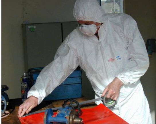
Use of tape and polythene sheeting to protect a work area before cleaning asbestos gaskets from a valve
