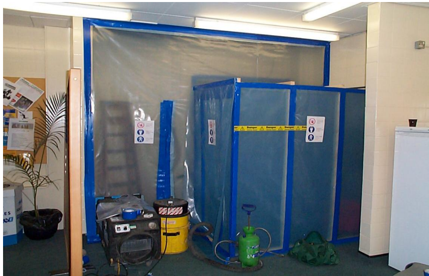
Fig X - Enclosure with 3 stage airlock, warning signage, transparent 500g polythene wall and unit to provide appropriate negative pressure. A H-Type vacuum is available for decontamination within the 3-stage airlock and a garden sprayer with PVA solution is on standby for any unforeseen release of asbestos fibre outside the enclosure
